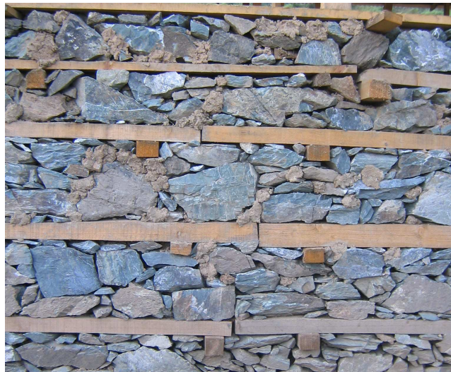
Figure 5. Common defects in modern bhatar constructions: poor connection between timber elements, poor alignment and connection of beam laps, and lack of through-stones.
